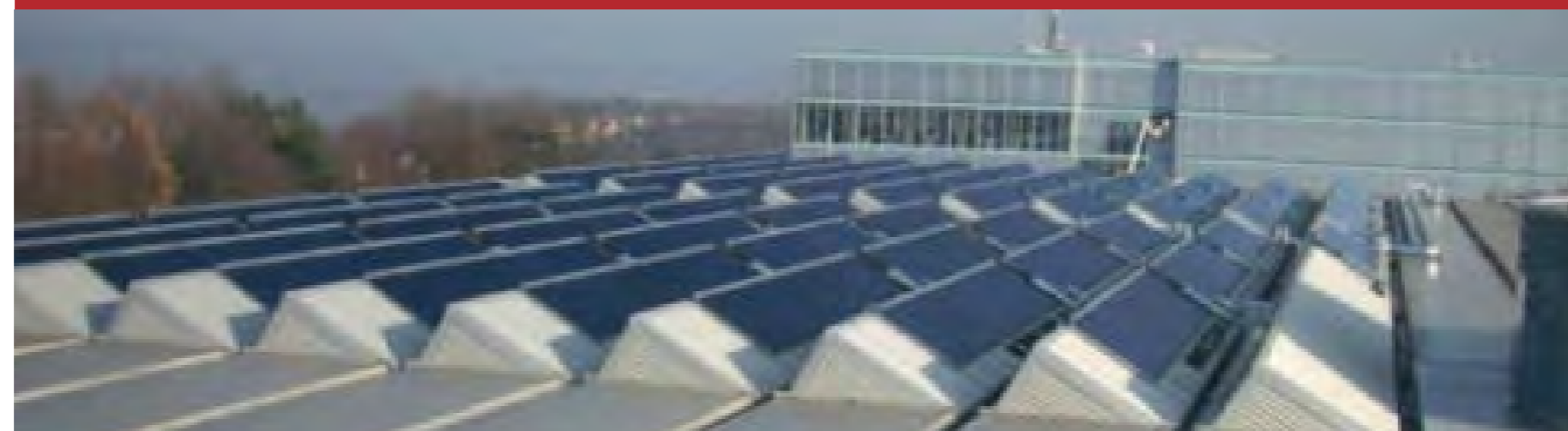
FIGURE 58: SOLAR THERMAL COOLING AND HEATING, ESSLINGEN, GERMANY SOURCE: SOLARSERVER
