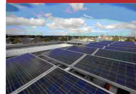
FIGURE 7: SOLAR PV, SURRY HILLS LIBRARY
