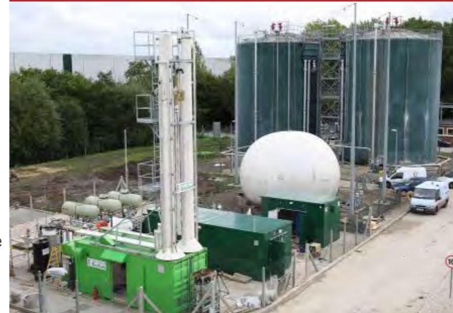
FIGURE 79: DIDCOT SEWAGE TREATMENT PLANT RENEWABLE GAS GRID INJECTION, OXFORDSHIRE, UK SOURCE: CNG SERVICES
