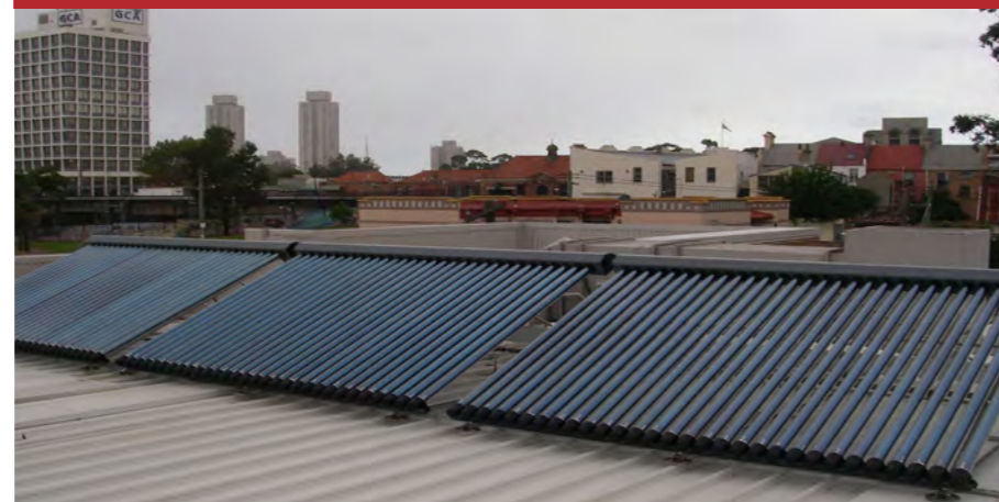
FIGURE 56: SOLAR THERMAL HOT WATER, REDFERN COMMUNITY CENTRE, SYDNEY SOURCE: CITY OF SYDNEY
